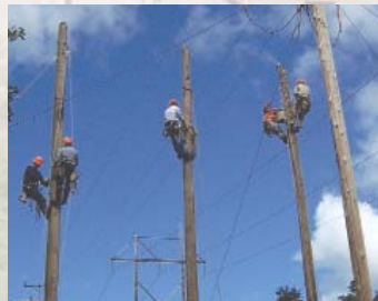
Line crews from throughout New York's Eastern Division replaced and repaired 6.4 miles of transmission line through mountainous terrain from Chestertown to North Creek, N.Y.
