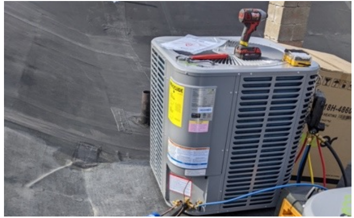
National Grid installed Ecoer electric heat pumps to replace McSwiggan's existing HVAC system. By transitioning from natural gas to electric, McSwiggan's will be able to reduce greenhouse gas emissions while operating more efficiently.
