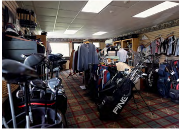
Pine Haven Country Club partnered with National Grid to install more efficient heat pumps and quieter air conditioning at Pine Haven Country Club’s pro shop.
