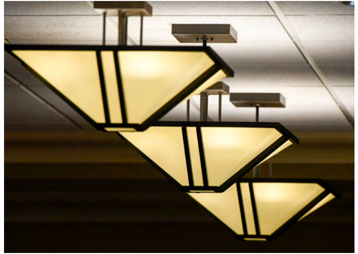
The lighting retrofit project took every room into consideration. The dining room, for example, switched from lights facing down to up so they could be diffused and increase guest comfort.
