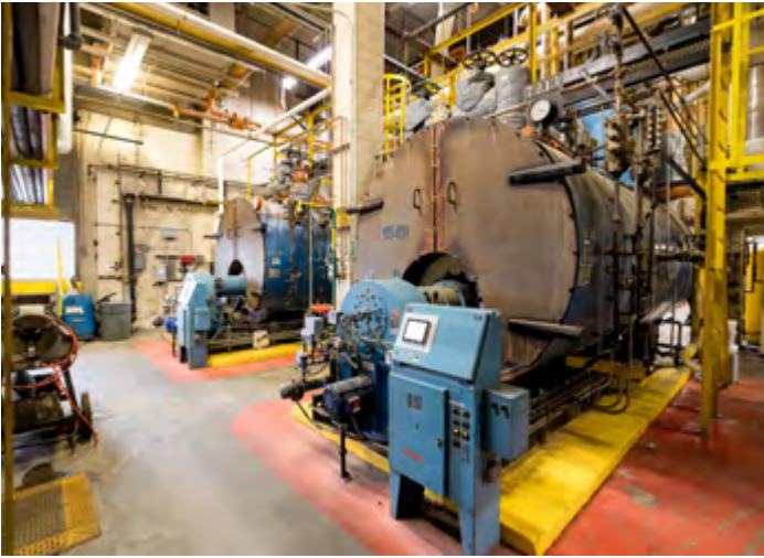
The boilers at Glens Falls Hospital normally run on natural gas, but during an event, can be switched to a backup fuel oil to alleviate strain on the gas system.
