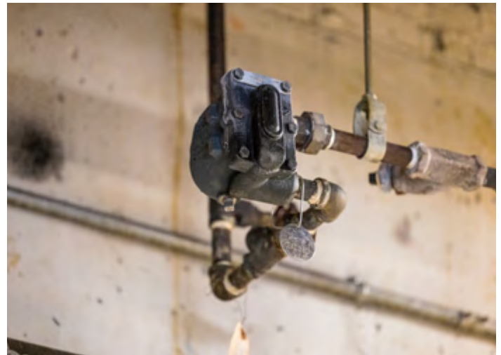
Glens Falls Hospital used National Grid’s energy-efficiency programs to conduct a steam trap survey, which led to the replacement of steam traps and significant annual energy savings.
