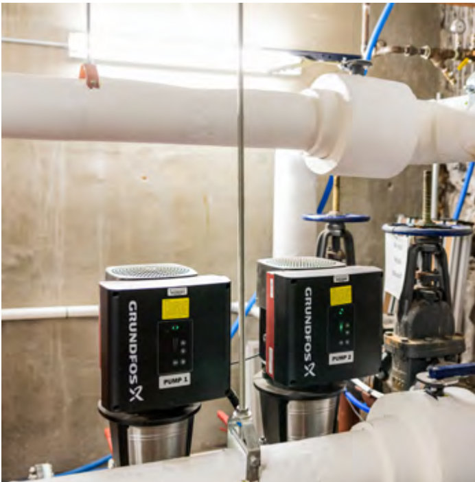
Some of the energy-efficiency projects at Glens Falls over the years included the installation of eight water booster pumps and LED lighting.
