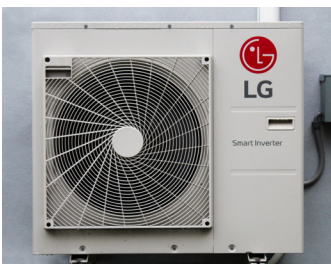
Safe Harbor installed two LG hyper-heat, multi-headed, heat pump systems in the studio.
