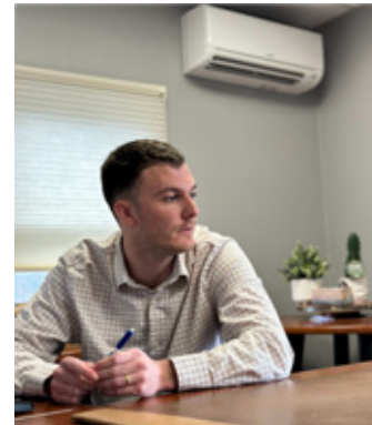
O'Connor installed two Mitsubishi hyper-heat, multi-headed, heat pump systems throughout offices and the main floor.
