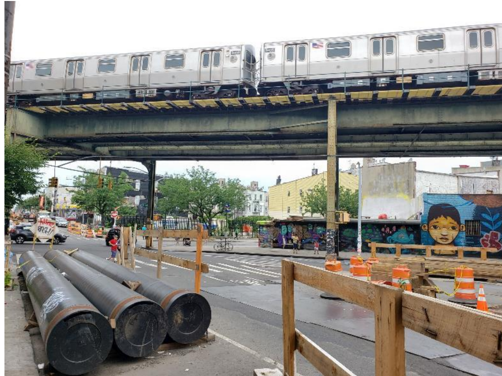
Metropolitan Reliability Infrastructure Project – Brooklyn, NY
